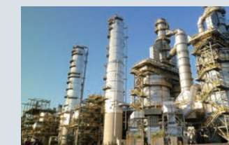
Para-xylene production facility
