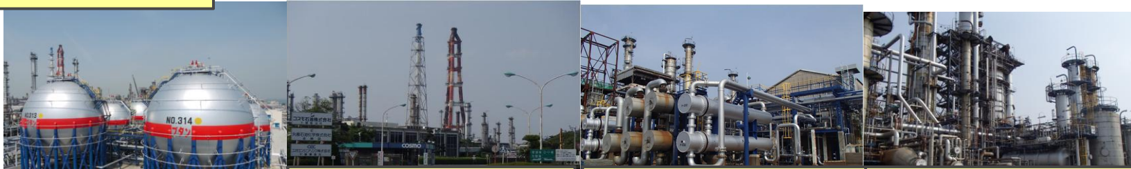
Newly installed LPG tanks
