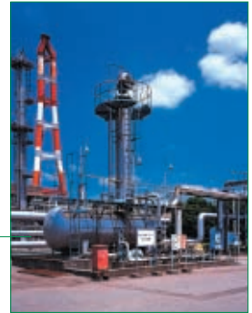
Hydrocarbon vapor recovery unit
